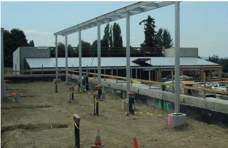
CNG Equipment Racks – Foreground BMF Building – Background
