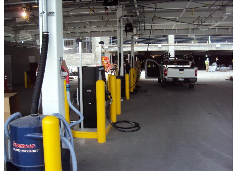
RCF QTA #1 Fuel Dispensing Equipment
